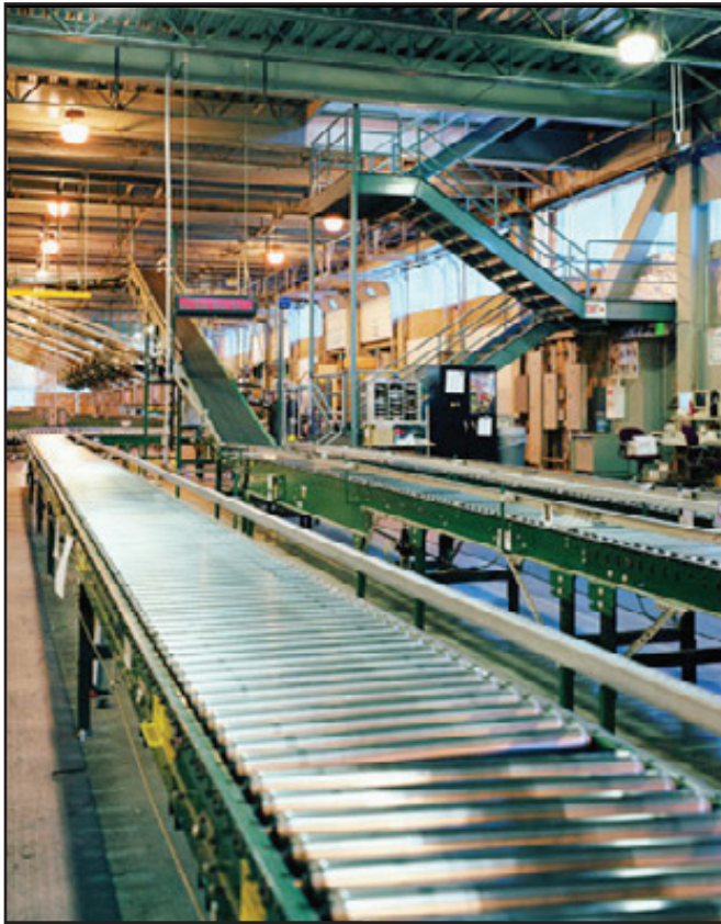
Figure 1 AC motors powering a BDLR conveyor
